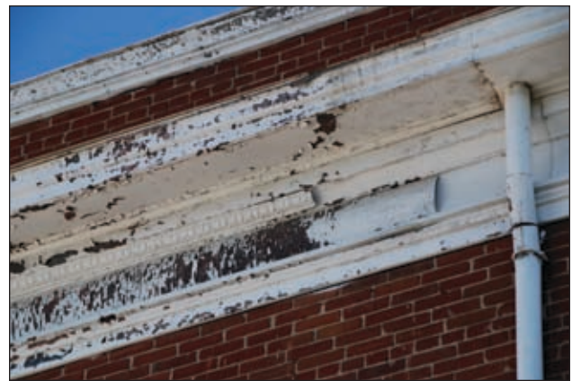
A good paint job would improve the architectural detail, and overall image of this site.
