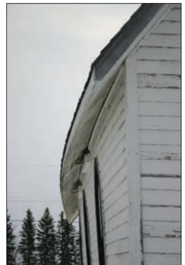
Bowing of an exterior wall, likely due to foundation issues, will eventually collapse if not repaired.
