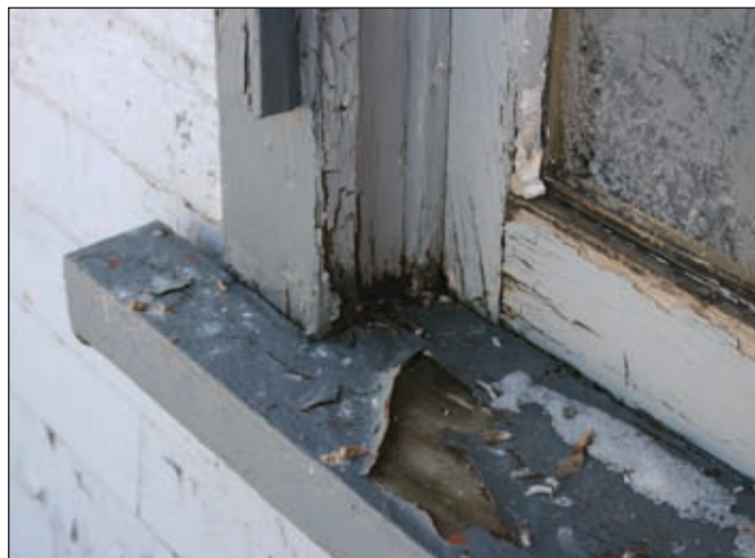
Water sitting on the sill has caused the paint to flake and the wood to deteriorate. The window sash and frame will have to be repaired with epoxy, or replaced depending on the severity of the rot.
