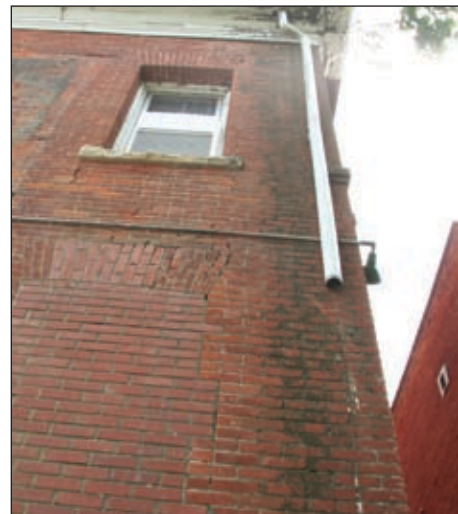
The missing downspout has created a build up on the exterior wall. Cleaning may do more damage, so it may be better to just leave it there.
