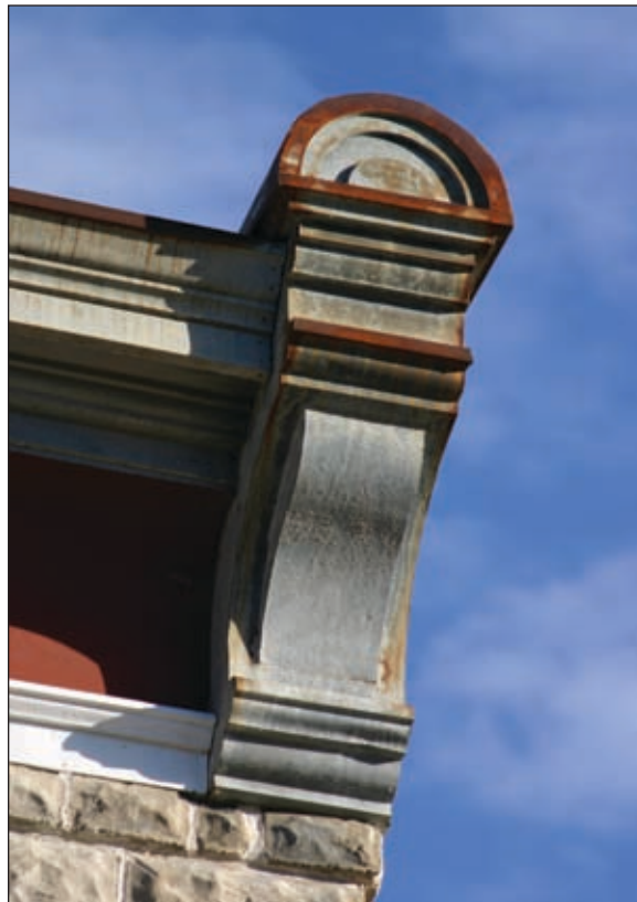
This eave bracket needs to be painted to prevent further deterioration by rust.
