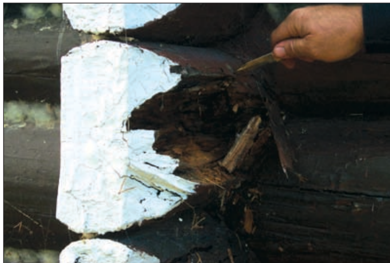
This log has been damaged by water. Investigate the source of the water and address the cause of deterioration before replacing the log.
