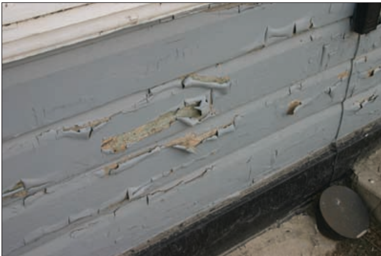
Peeling or flaking paint is often a sign of heat or water damage. The best treatment is to remove as much loose paint as possible; identify if the existing layer is oil-based or latex paint; prime with appropriate exterior primer; and apply a fresh coat of paint.
