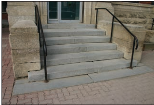
These steps need to be inspected as the freeze/thaw cycle is causing some lifting. A mason may have to re-level them.
