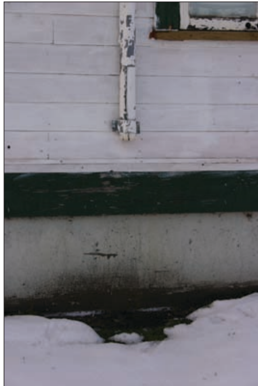
With a missing downspout and inadequate grading, water is allowed to collect at the base of the building and can cause significant damage.
